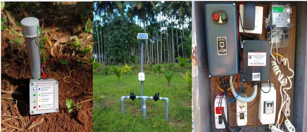
Smart Irrigation Control
